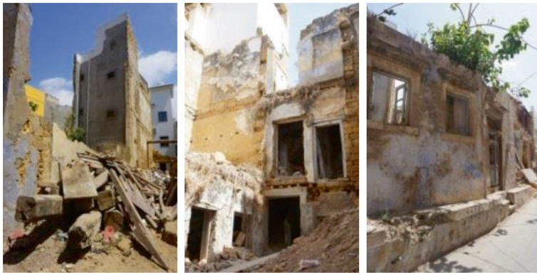
Figure 2: Deteriorating heritage structures of Diu Town (Source: Meggi, A. 2017).
